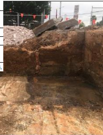
Northern UPSS excavation pit north wall, showing water ingress
